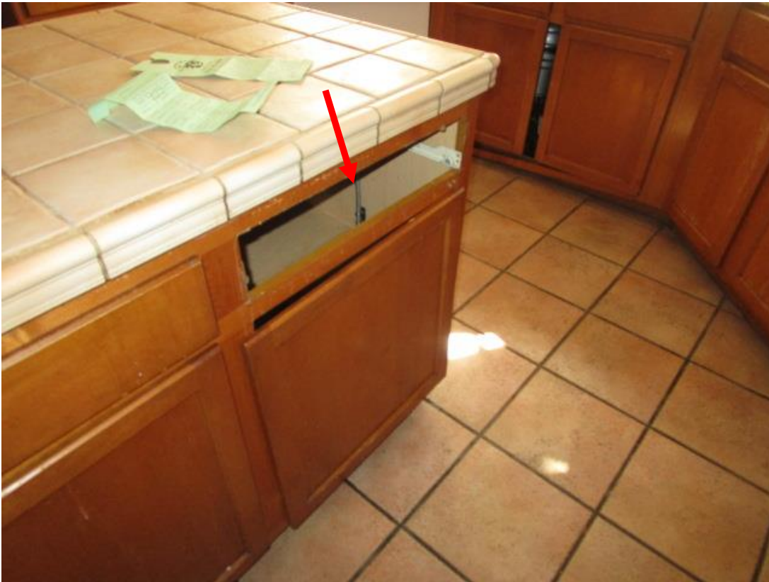
Broken kitchen cabinet & missing drawer needs to be serviced
