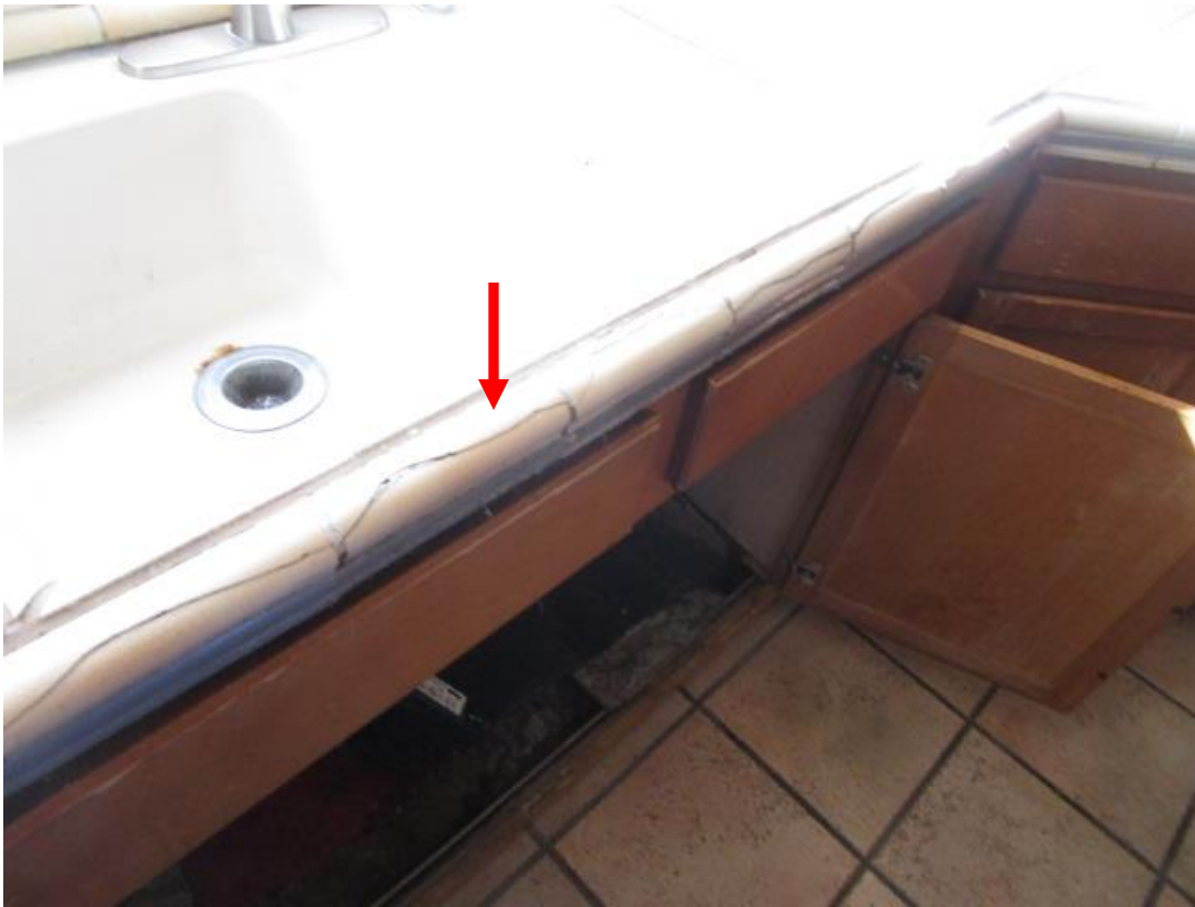
Crack in counter top needs repair
