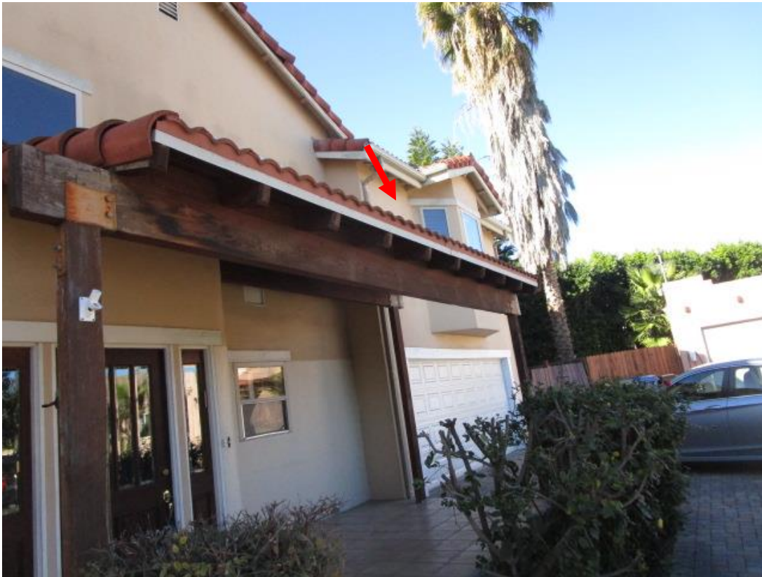
Missing gutter and Downspouts needs to be serviced
