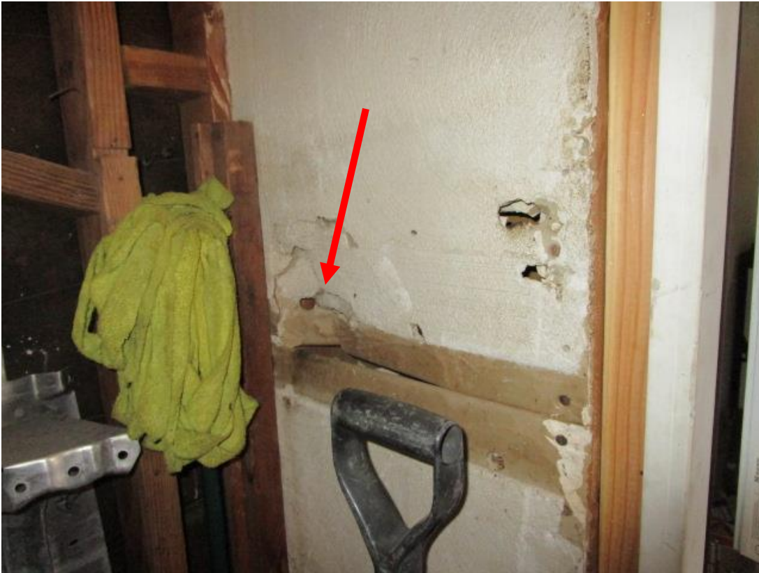
Crack dry wall in garage needs repair
