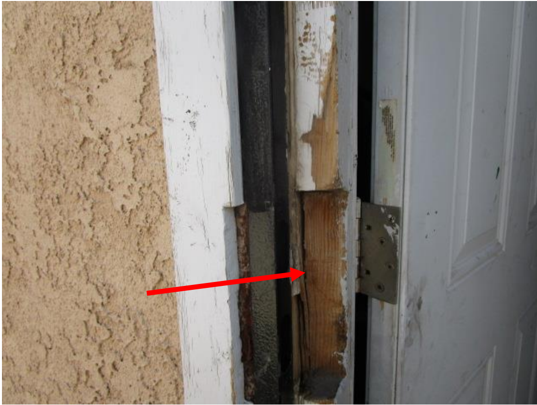
Damage frame door needs to be serviced
