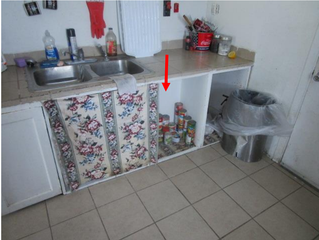
Missing cabinets door in kitchen needs to be serviced
