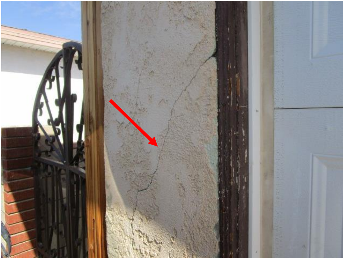
Crack stucco needs repair
