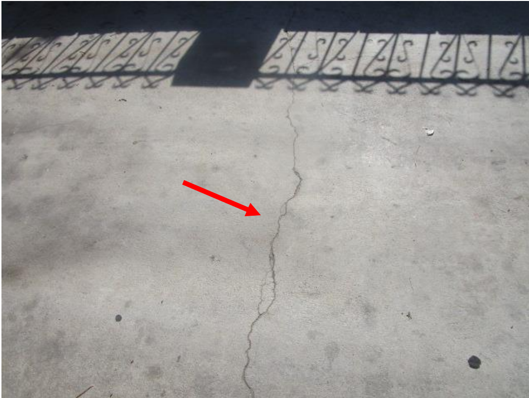
Crack on concrete floor in drive way needs repair
